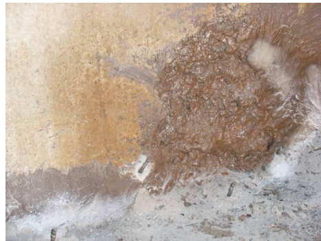
Picture 4. Water stops leaks with quick hardening materials
