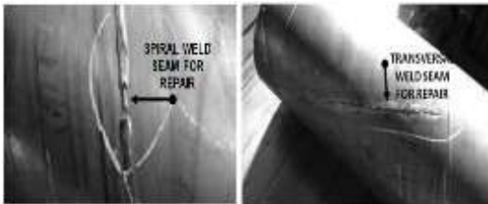
Fig.2. Pipes with defects in weld seam
